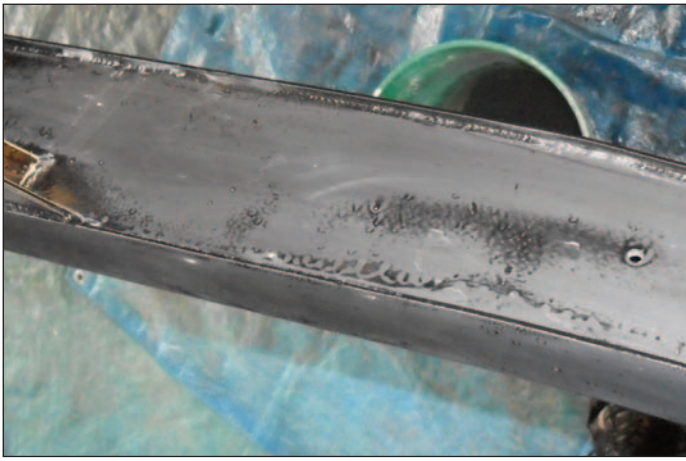
ABOVE: Here you can see an area inside the boxed section of the chassis rail where the RustSeal paint sagged from applying too much too quickly. Make sure you rub such areas right out flat again before top coating.
